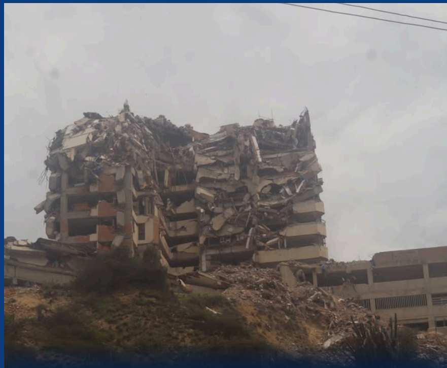
A tower sheared off
