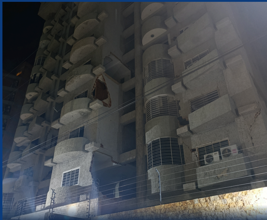
Families still behind open walls
